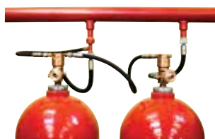
Fire Suppression Agent Cylinders
