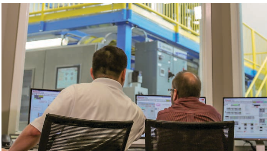
FIG. 1. A properly designed and certified F&G safety system provides information to the PCS to enable operations to consider both process and environmental conditions in a hydrocarbon processing facility.
