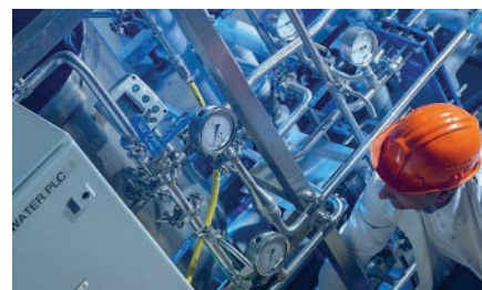
FIG. 2. Industrial processes, usually controlled by a PCS, must also be protected by an F&G safety system that can detect and provide a warning of hazardous conditions.
