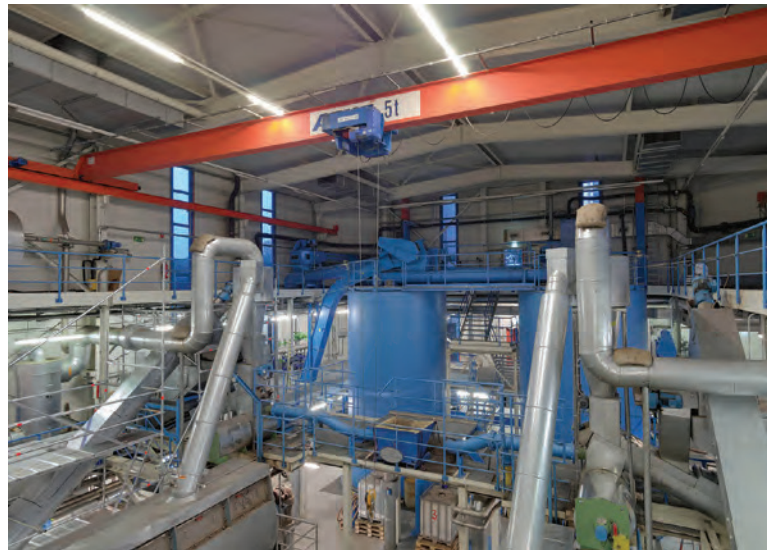
Biosolids dewatering is one wastewater treatment area specifically called out in NFPA 820 for fire protection that includes smoke detectors.
