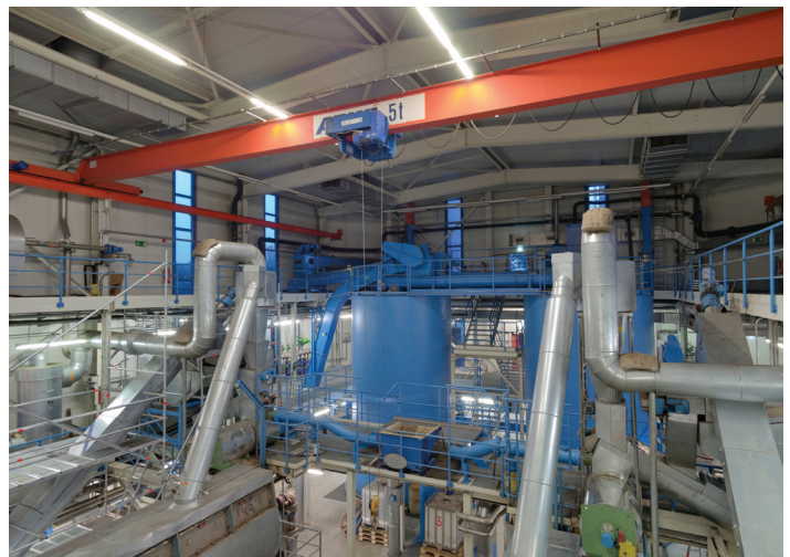
Sludge dewatering is one of the wastewater treatment stages specifically called out in NFPA 820 for fire protection including smoke detectors.
