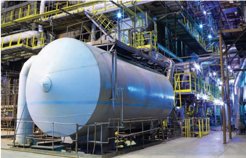
FIGURE 2. Hazardous areas in hydrocarbon processing plants are protected by life-safety gas detectors as part of a total risk-mitigation system.
